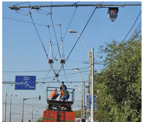
The High Wire Artists: Line crews install a switch on the new 4.3 km trolleybus extension in Bucharest, Romania. [Marian Andrei]
